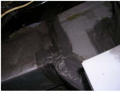
Inadequate insulation in the floor joist behind knee wall
