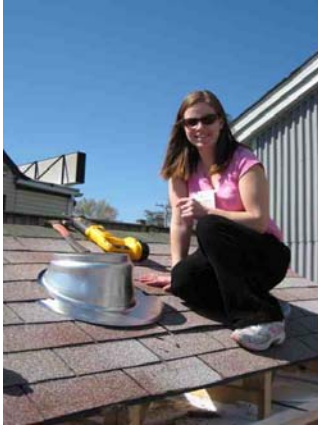
Green Building Institute Executive Director, Hannah Wood, helps install a Daylight Tube
